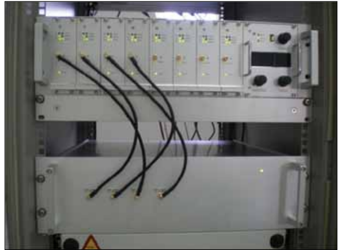
Figure 7. Front view of the IF processor (bottom rack) installed in the backend room below the FFTS.
